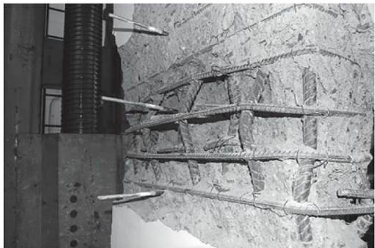
(c) Photograph of failed section
