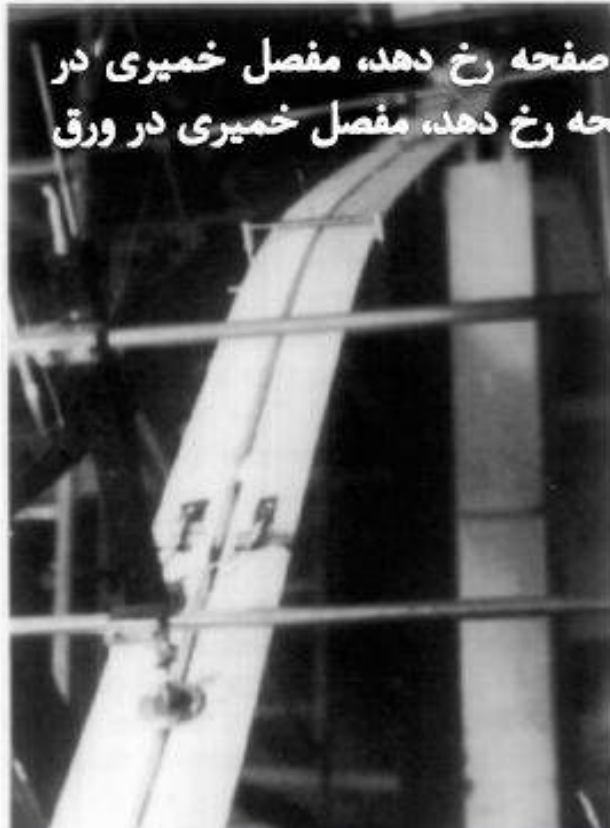
In-Plane Buckling of Bracing Members
