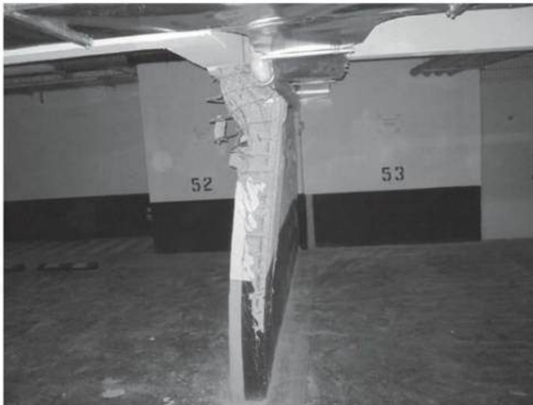
(a) 2010 Chile earthquake
