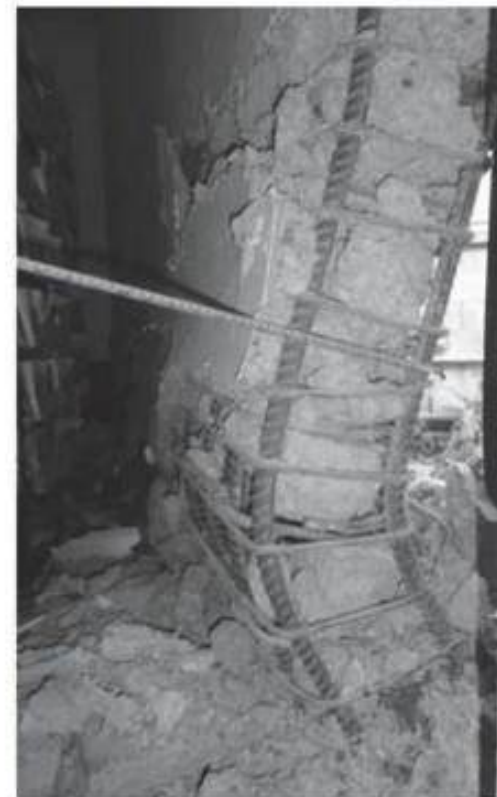
(b) 2011 Christchurch earthquake
