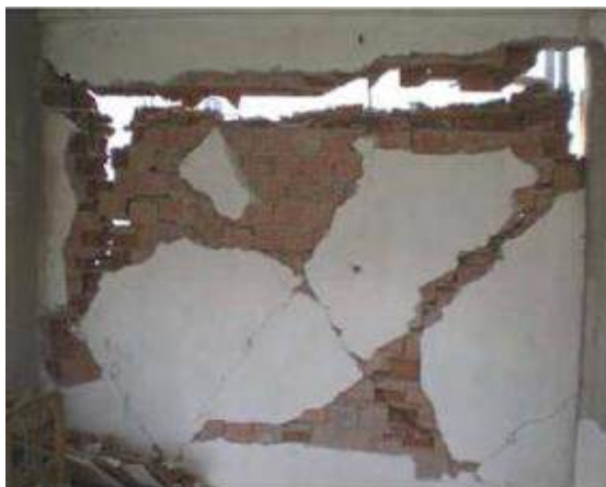
Kutahya Earthquake, Turkey May 29, 2011
