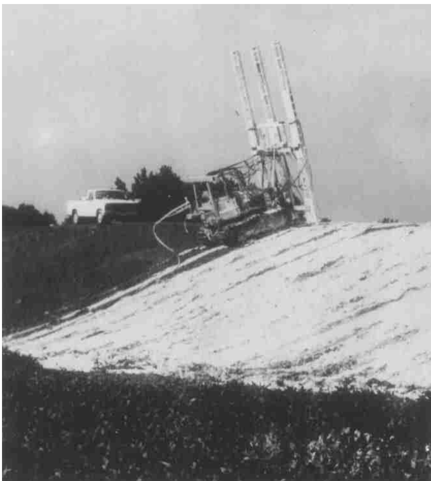
Figure 16.31 Pressure injection of lime slurry (Courtesy of Hayward Baker Inc., Odenton, Maryland)
