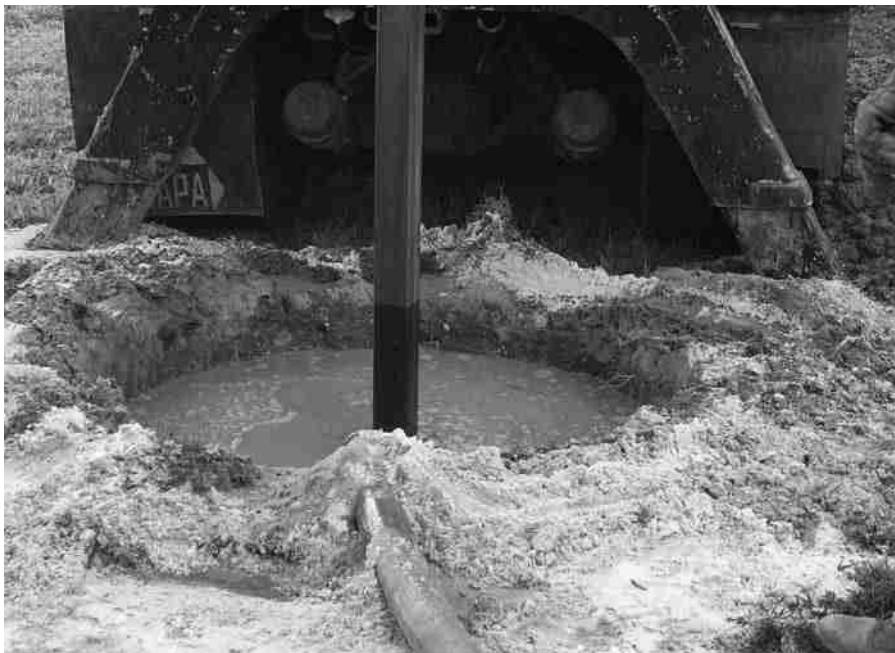
Figure 10.6 Drilled shaft construction using wet method (Courtesy of Khaled Sobhan, Florida Atlantic University, Boca Raton, Florida)
