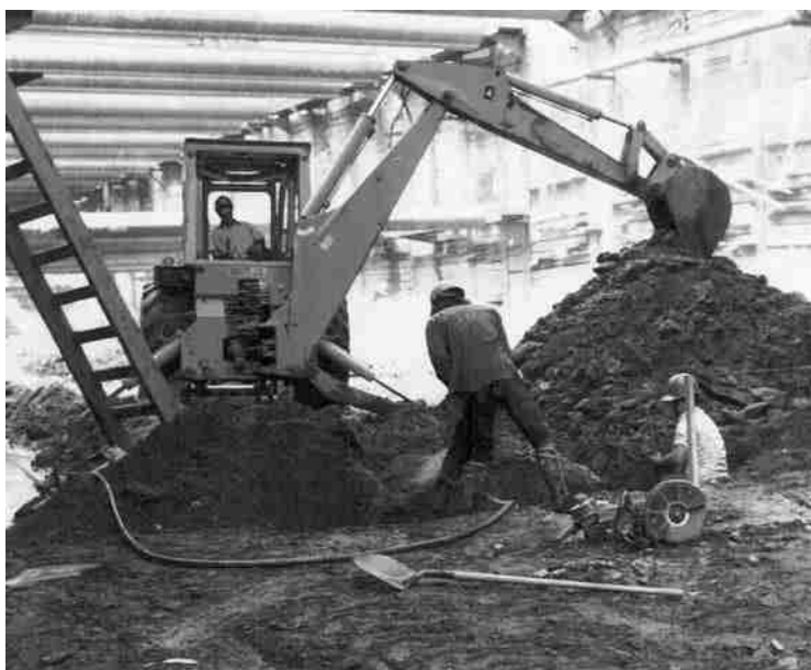
Figure 15.3 Braced cut in the construction of Washington, D.C. Metro, May 1974 (Courtesy of Ralph B. Peck)
