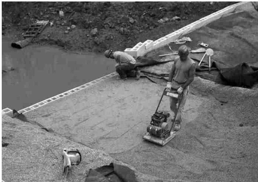
Figure 13.32 Construction of a geotextile-reinforced retaining wall (Courtesy of Jonathan T. H. Wu, University of Colorado at Denver, Denver, Colorado)
