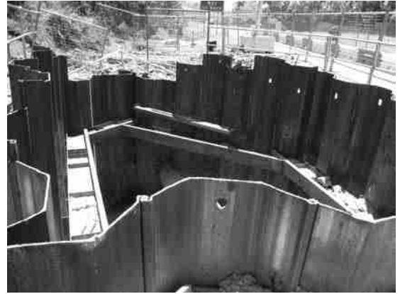
Figure 14.5 A small enclosure with steel sheet piles for an excavation work (Courtesy of N. Sivakugan, James Cook University, Australia)
