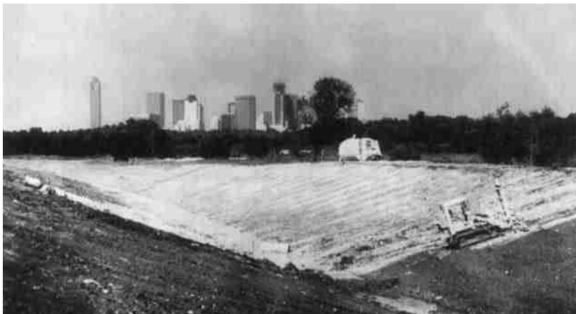
Figure 11.24 Slope stabilization of a canal bank by pressure injection of lime-fly-ash slurry (Courtesy of Hayward Baker Inc., Odenton, Maryland.)
