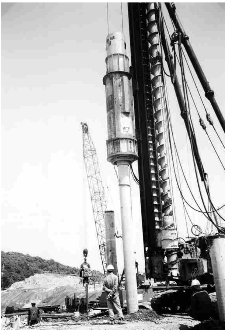
Figure 9.8 A pile-driving operation in the field (Courtesy of E. C. Shin, University of Incheon, Korea)
