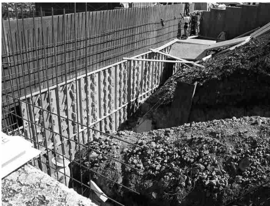
Figure 13.2 A cantilever retaining wall under construction (Courtesy of Dharma Shakya, Geotechnical Solutions, Inc., Irvine, California)
