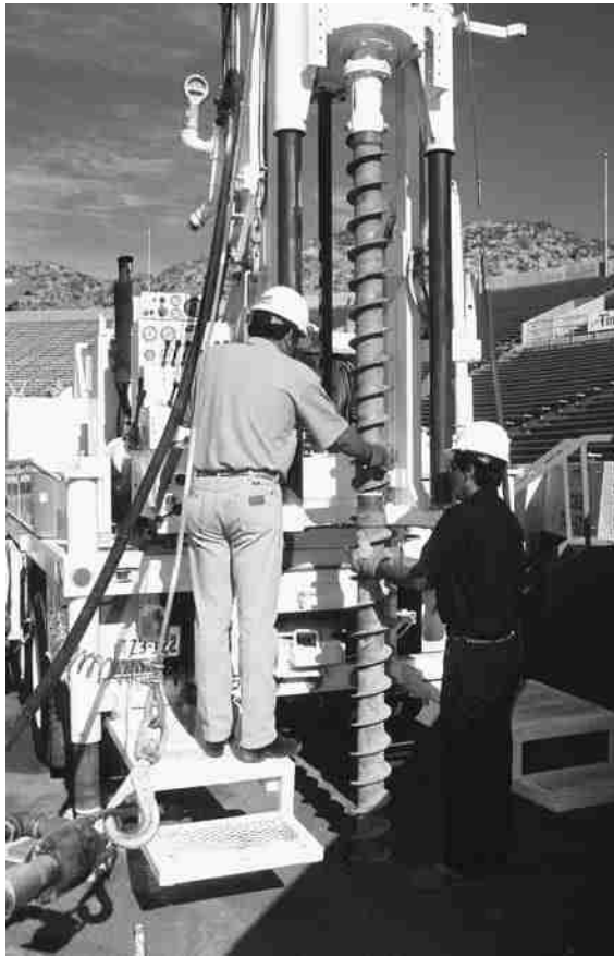
Figure 3.12 Drilling with continuous-flight augers (Danny R. Anderson, PE of Professional Service Industries, Inc, El Paso, Texas.)
