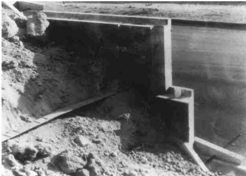
Figure 13.26 Metallic strip attachment to the precast concrete slab used as the skin (Courtesy of Braja M. Das, Henderson, Nevada)
