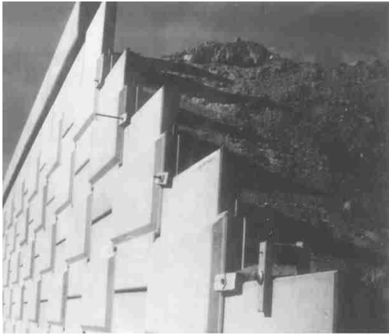
Figure 13.25 Another view of the retaining wall shown in Figure 13.24 (Courtesy of Braja M. Das, Henderson, Nevada)
