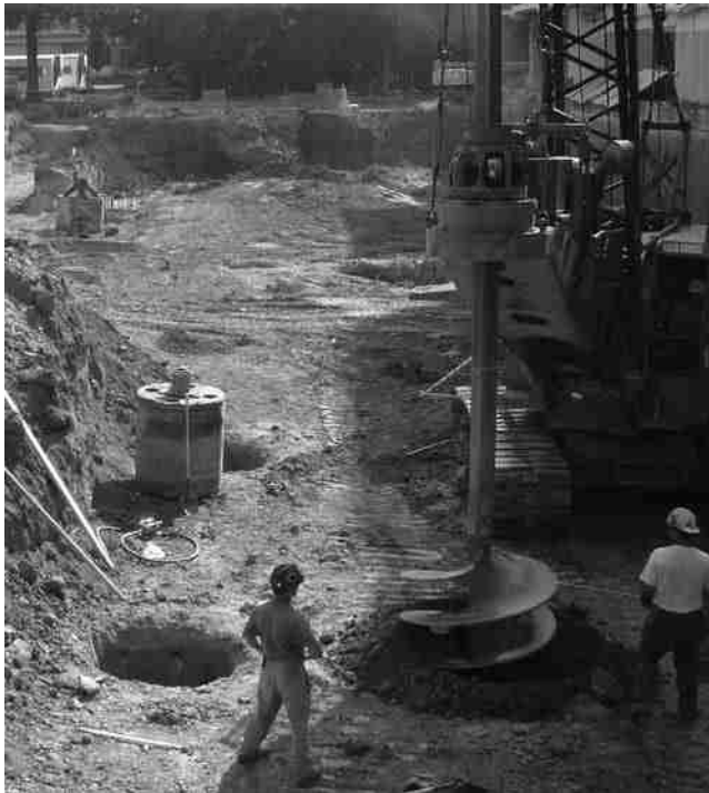
Figure 10.5 Drilled shaft construction using the dry method (Courtesy of Sanjeev Kumar, Southern Illinois University, Carbondale, Illinois)
