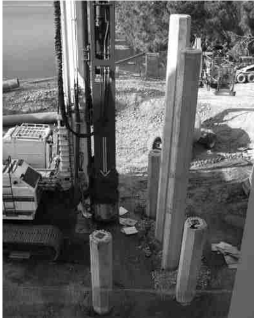
Figure 9.45 Driving of piles in a group (Courtesy of N. Sivakugan, James Cook University, Australia)
