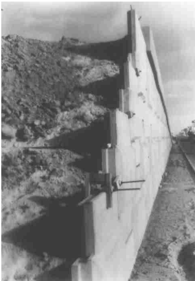
Figure 13.24 Reinforced-earth retaining wall (with metallic strip) under construction (Courtesy of Braja M. Das, Henderson, Nevada)
