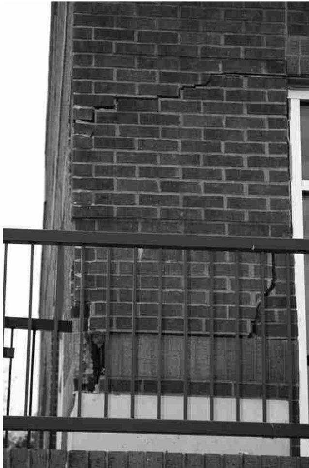
Figure 11.8 Cracks in a wall due to heaving of an expansive clay (Courtesy of Anand Puppala, University of Texas at Arlington, Arlington, Texas)
