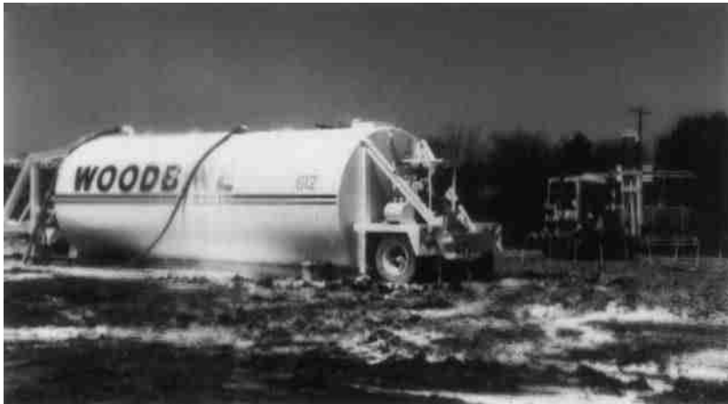
Figure 11.23 Pressure injection of lime slurry for a building pad (Courtesy of Hayward Baker Inc., Odenton, Maryland.)
